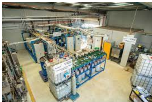
Neometals vanadium recovery from slag plant
