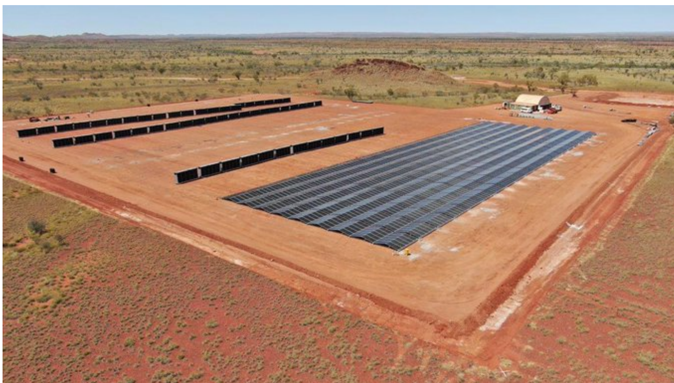
Calidus Resources new solar and battery farm at the Warrawoona Gold Mine, WA.
