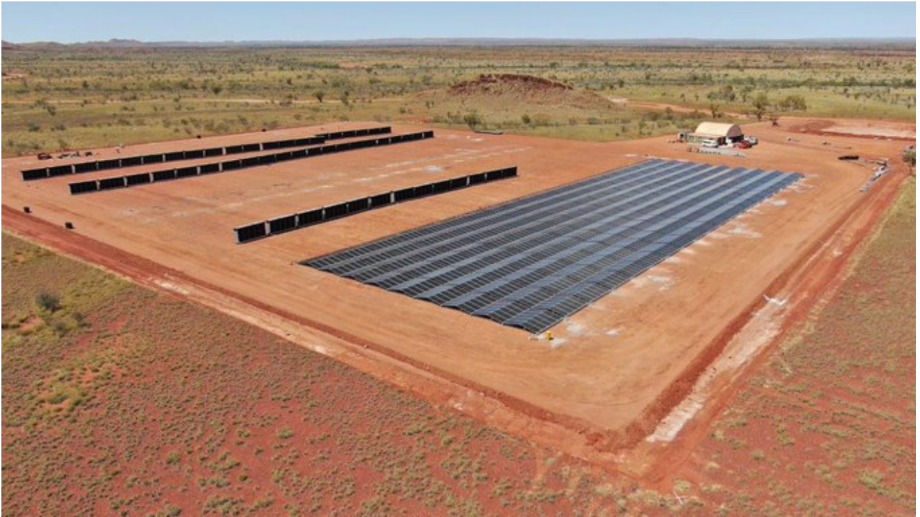
Calidus Resources new solar and battery farm at the Warrawoona Gold Mine, WA.
