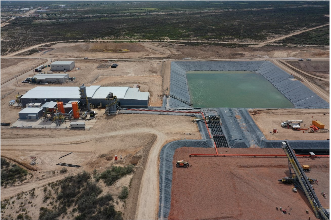
Orla Mining heap leach pad, Solution pond, and Merrill-Crowe plant
