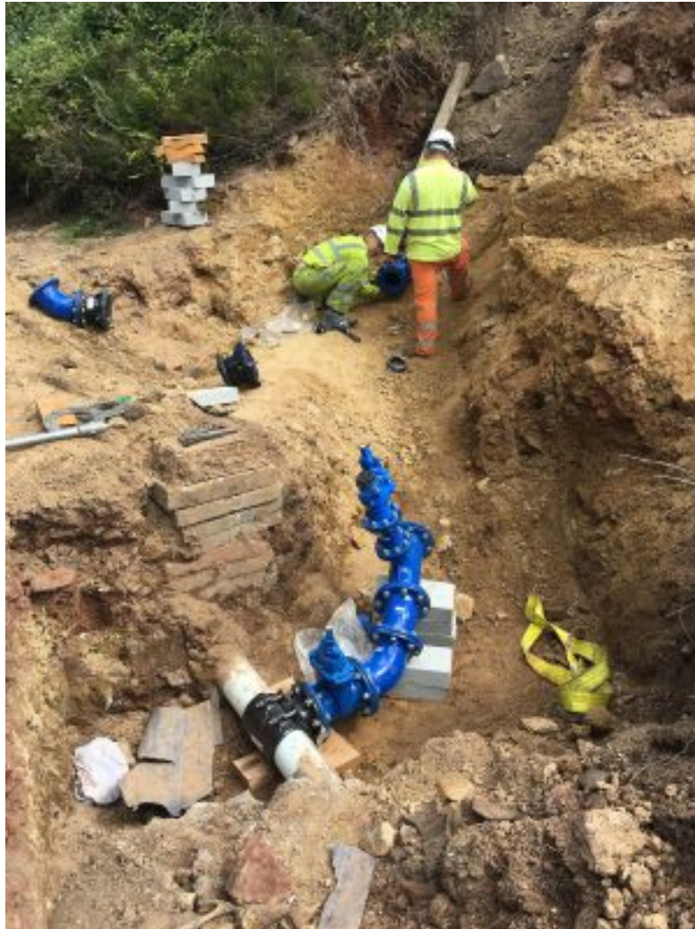
Cornish Metals water treatment works at South Crofty
